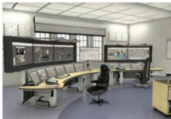
FIGURE 3. Operators at a modern control room monitor both the operation of the process as well as the safety and security of the plant
