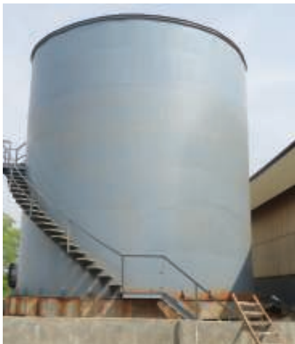
FIGURE 4. Proper care must be taken when executing hot works in the presence of sulfuric acid storage tanks
