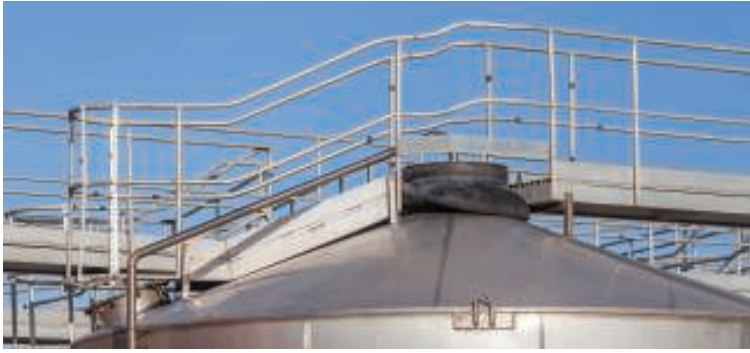
FIGURE 3. A metal catwalk on the roof of a storage tank provides some protection for workers, as it is unsafe for personnel to walk directly on a tank's shell
