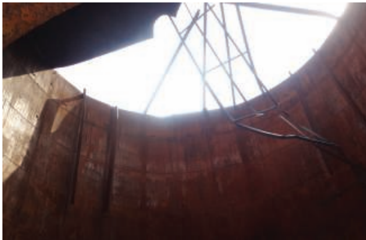
FIGURE 5. The same tank from Figure 4 was badly damaged after its roof exploded due to hot work on the roof and the formation of hydrogen gas inside the tank while the tank was in service
